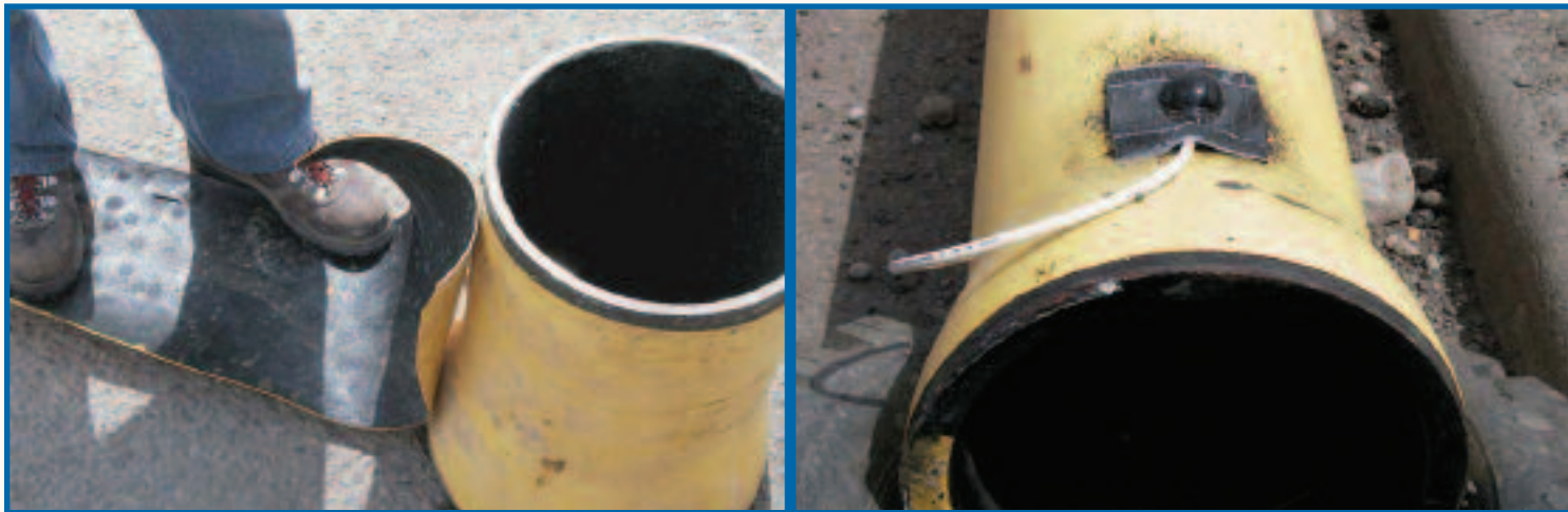
Figure 7: "Yellow-Jacketed" ductile iron (YDI)
