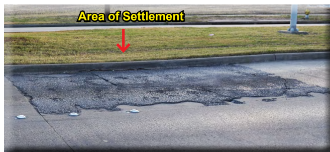
Leaking joints damage infrastructure.
