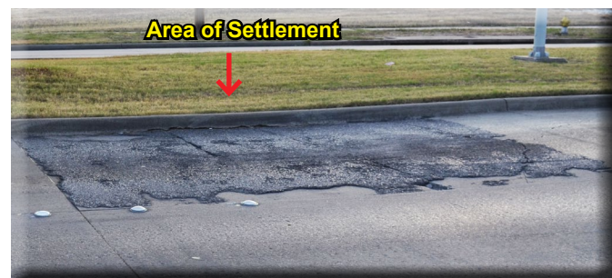
Leaking joints damage infrastructure.
